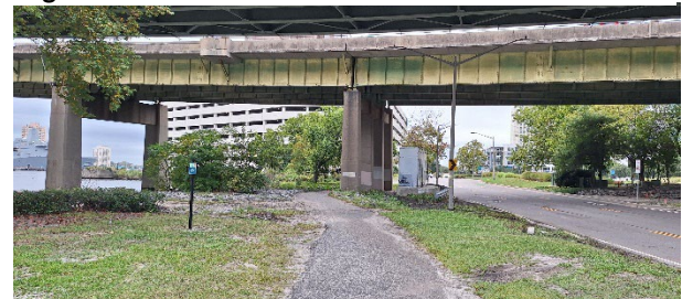
Figure 2 Washout after rain event
